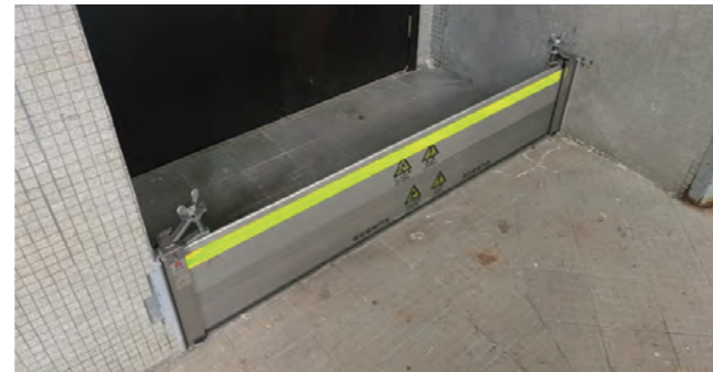
Flood Gate at Regal Airport Hotel
